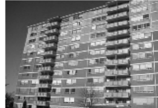
Photo 3: Exposed Frame. The bad news is that we have built lots of these. The good news is that they are easy to fix by recladding them with exterior insulation.
